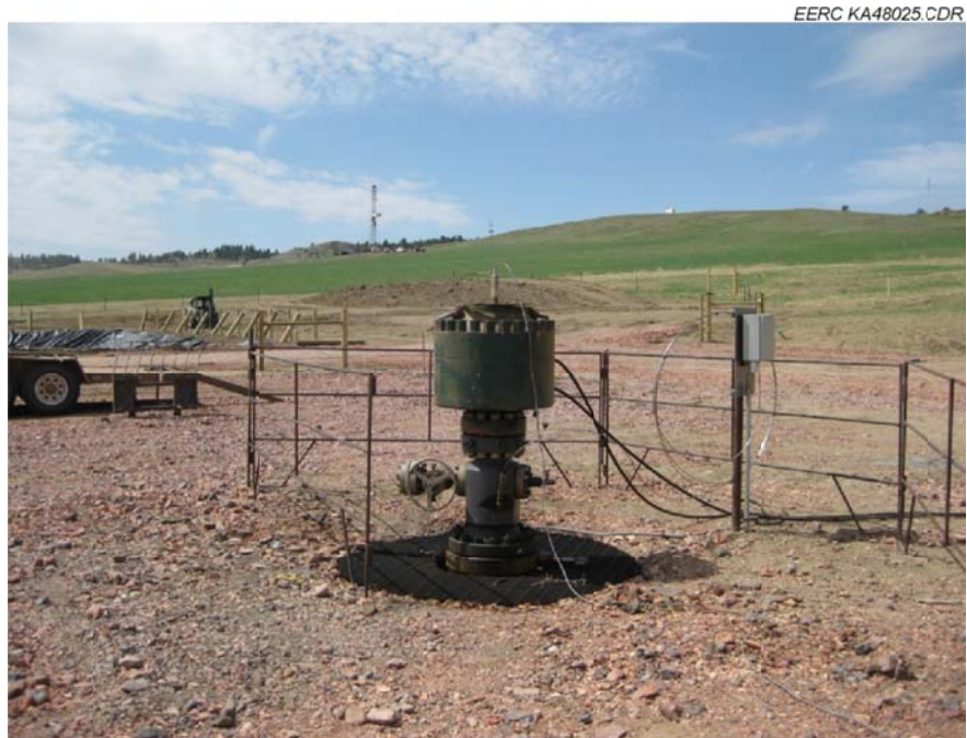
Figure 7. Bell Creek monitoring well 05-06 OW with a 50-level removable seismic receiver array hanging in it. The wire coming out of the wellhead is a fiber optic cable carrying 150 channels of data to the nearby recording trailer (May 2013).
