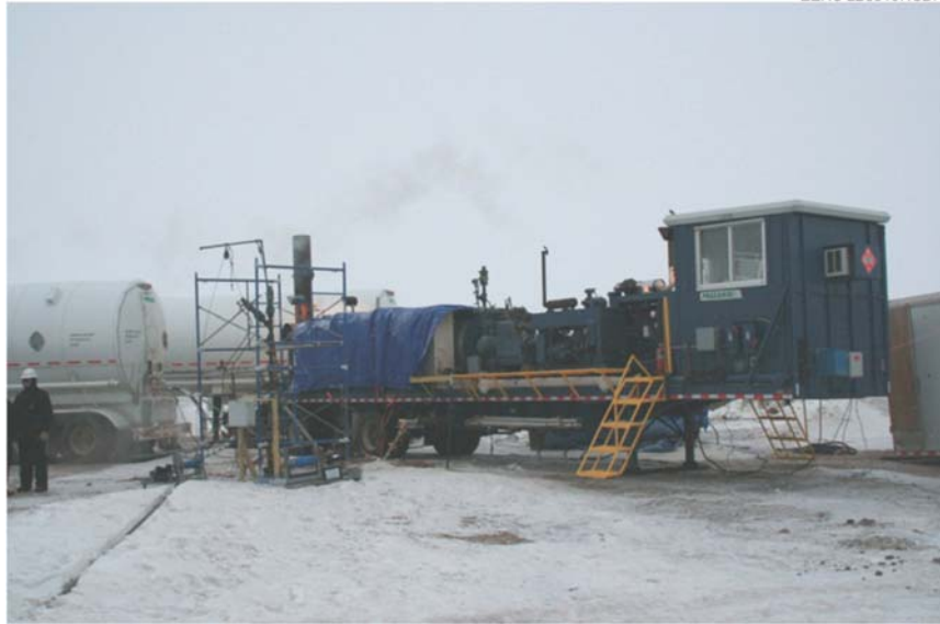
Figure 9-1. Site photo of pump skid and CO 2 storage tank.
